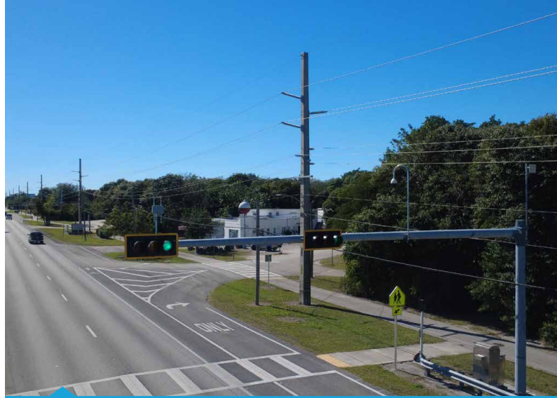
Traffic Signal Along U.S. 1/Overseas Highway
