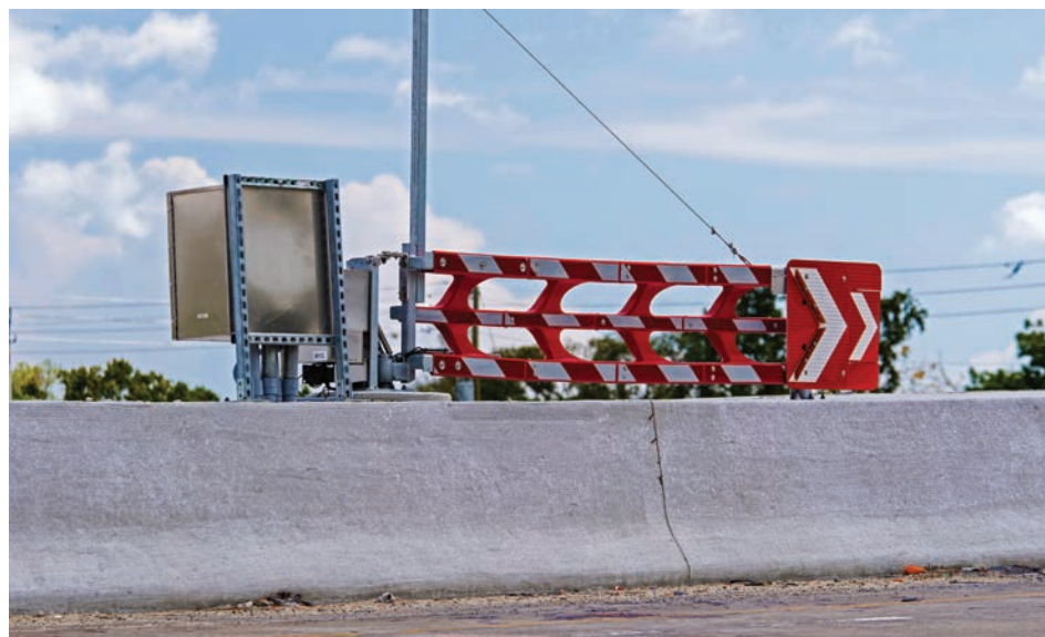
I-95 EXPRESS LANE ENTRANCE WARNING GATE
