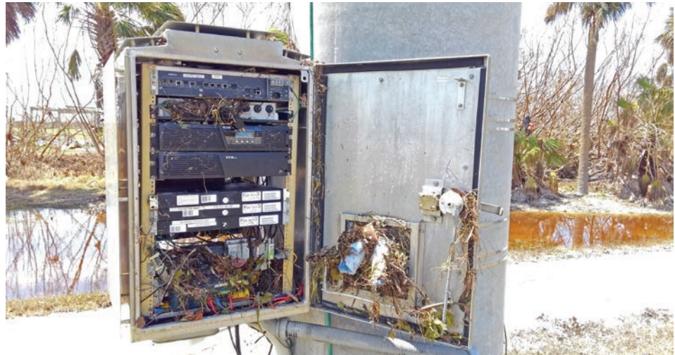
ITS CABINET IN FLORIDA KEYS AFTER HURRICANE IRMA
