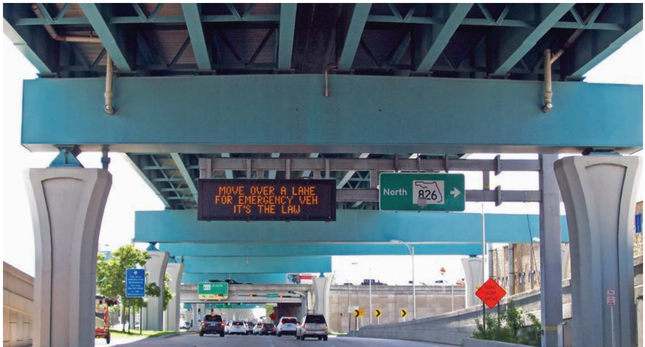
ARTERIAL DMS UNDER THE NW 25 STREET VIADUCT
