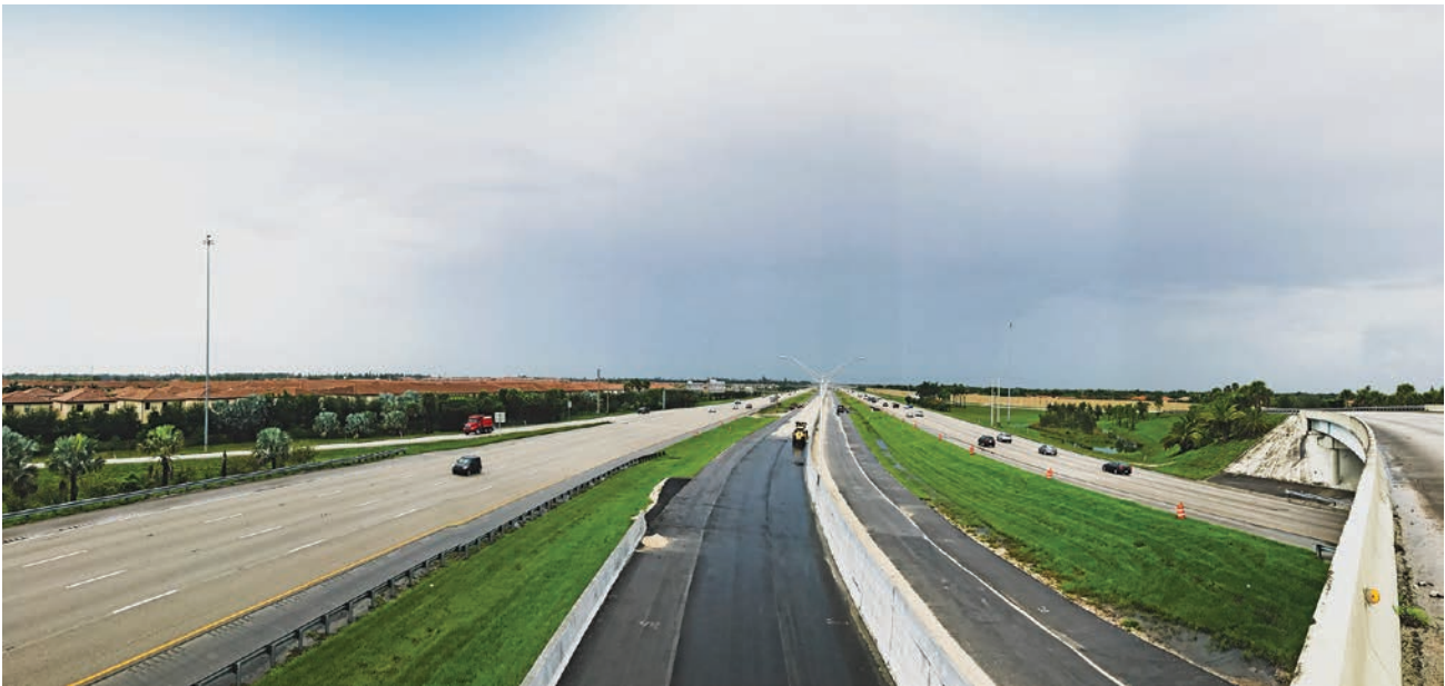
TOP LEFT: ARTERIAL OPERATIONS IN THE FLORIDA KEYS; TOP RIGHT: TOLL AMOUNT DMS RETROFIT FOR 95 EXPRESS ABOVE: CONSTRUCTION OF I-75 EXPRESS LANES
