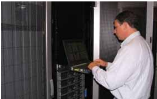
System Availability of ITS Equipment reached 97% during FY 2007/2008
