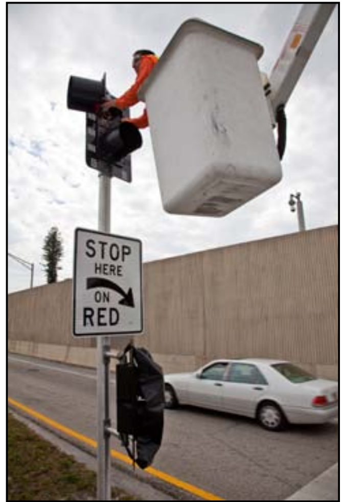
Maintenance crew works on a ramp signal along I-95 in Miami-Dade County.
